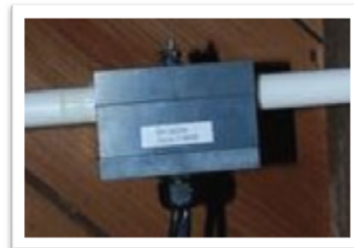
Water Flow Meter
